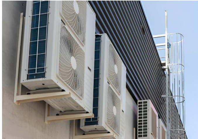
Heat pump for space heating
