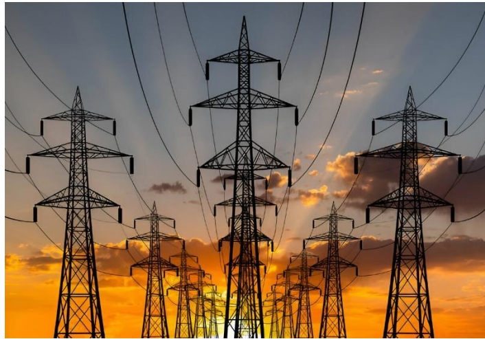
Extensive power grids used for renewable incorporation
